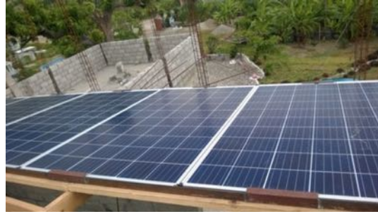
Fig. 12: The center of the six 260W panel array installed during the March 2017 trip to Coteaux, Haiti. The installation employs a novel racking design created by local welders with galvanized steel studs that allows easy removal in the event of another tropical storm/hurricane.
