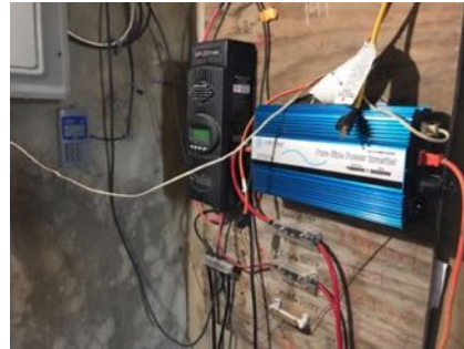
Fig. 6: The power electronics of the 1.5 kW Provisional PV system installed during the first trip to Coteaux in March of 2017. The inverter will be replaced by two larger Outback inverters in the full system, while the Outback charge controller shown is transferable to the full system.
