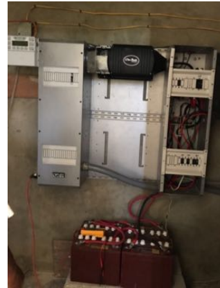
Fig. 15: The operational Outback system installed during the June 2017 trip. The final system will consist of a second inverter, and two more charge controllers attached to the right side of the electrical enclosure. Seen is the 7 kWh lead acid battery bank which will be replaced by the 20 kWh LFP bank in the Fall of 2017
