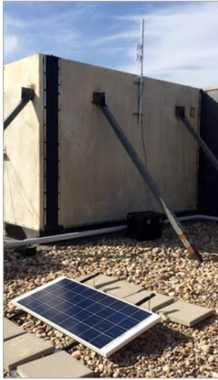
Figure 12: The installation at the Space Sciences (SPSC) building. Visible is the 140W PV Panel, the mast with two DLB Propeller 5s attached, and the electronics enclosure slightly obscured by the wall shadow. Two Propellers are colocated with a second Raspberry Pi to add more load to the network without the need of additional power electronics.
