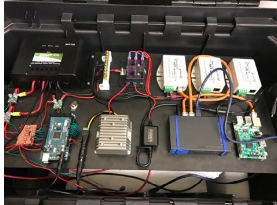
Figure 7: The array of electronics found at each client station. Starting in the upper left and moving clockwise there is: LFP Charge Controller, DC Bus, two 24V PoE Injectors, one 48V PoE Injector, Raspberry Pi 3, Linksys five port Switch, Buck Converter, Voltage Regulator, Arduino, Circuit Board, and three Current Monitors.
