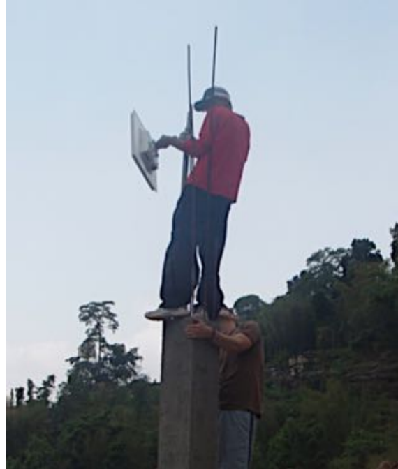
Figure 2: Binod Bidari of the Nepal Wireless Networking Project (NWNP) working with University of Colorado at Boulder students on a WiLDNet installation in the Ilam District in eastern Nepal in June of 2009. Binod is aligning a Wi-Fi Long Distance transceiver to form a point to point connection with the village of Namsaling that lies on the far (eastern) side of the Mai River.
