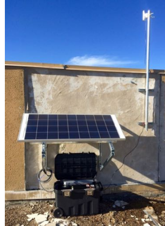
Figure 13: The South Complex installation, where the panel, electronics enclosure, and mast/radios are clearly visible. This client station is located 3.89 km southeast of the EC Tower base station.
