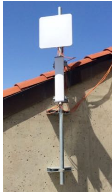
Figure 5: The Base Station mast on the south side of the Engineering Center Tower. Shown are a Ligowave DLB 5-90-17 with a 90 degree sectoral (lower) for point to multipoint transmission and Ligowave PTP 5-N-23 long range point to point unit that will be used for longer (greater than 20 km) links.
