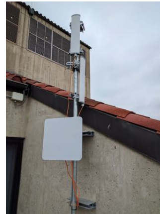
Figure 15: The north side of the EC Tower with two DLB 5-90-17s and a LigoWavePTP 5-23 installed. Installation location is the 8th floor of the Engineering Center, atop a mesa, allowing a commanding view for 40+ km to the north.
